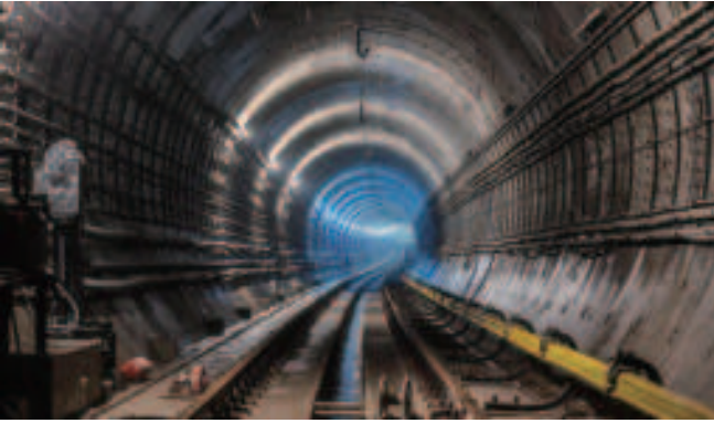
Subway water drainage
